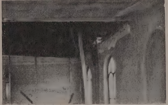
Broken roof truss at Bolton Elim Church. Supporting beams hold up the roof.
