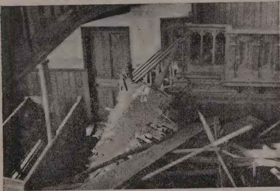
Part of fallen ceiling in Bolton Elim Church.
